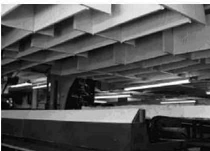
More than 600 Polywrapped Ceiling Baffles reduced overall noise levels by 8 dB(A) in this wood working facility.
