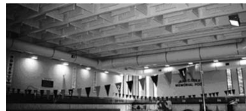
In addition to reducing reverberating noise, the durable, chemical resistant and water-tight construction of Sanitary Baffles makes them suitable in difficult environments such as this swimming pool.
